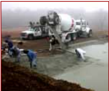
Dec. 11: 'Twas a misty moisty morning for pouring the concrete floor, but it was ideal weather for the job, completed in just two hours.
