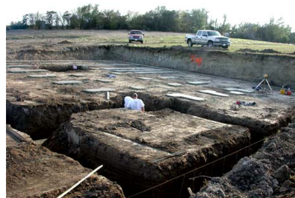
The real groundbreaking began on October 16 when Rob Roberts of Mid-Nebraska Land Developers donated excavation services. Here, the concrete contractor is pouring the foundation footings.
