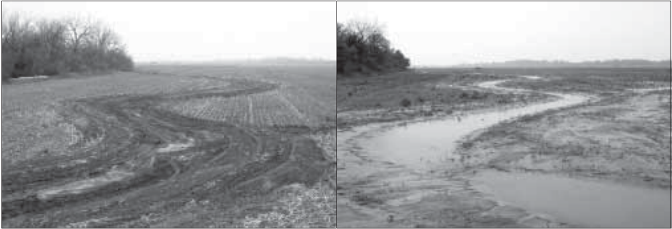
In lowland areas, such as the Platte River valley, excavating fill material can create a shallow water wetland that can be seeded to a marsh or wet-mesic prairie community.
